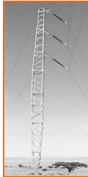
Plate 2.3: Example of a single pole steel lattice pylon.
